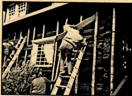
BEFORE AND AFTER: Volunteers from the West Seattle Kiwanis Club strip newer siding from the south wall of the cabin in January. See page 2 for faces and names.
