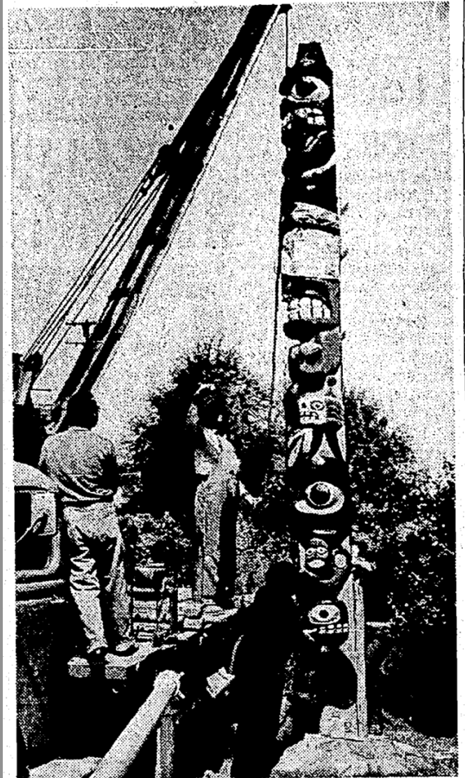
IN PLACE AGAIN: Park Department workmen today replaced a 100-year-old totem pole in West Seattle's Belvidere Park on Admiral Way after several weeks of "major surgery" to repair the landmark. The 35-foot tourist attraction, painted in bright new colors, weighs about 350 pounds. Jon Abrahamson, carpenter foreman, mixed a compound to seal deep cracks in the weathered pole. The Park Department had been uncertain whether the pole could be saved when it was removed March 27 for the repair project.
